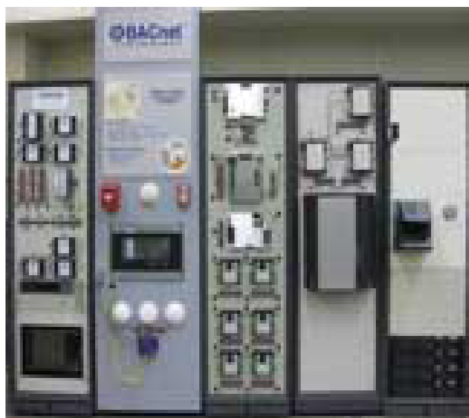
Embedded Intelligence in Buildings
